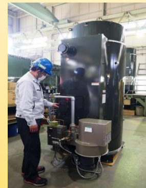
Gas Boiler (372 kW)
